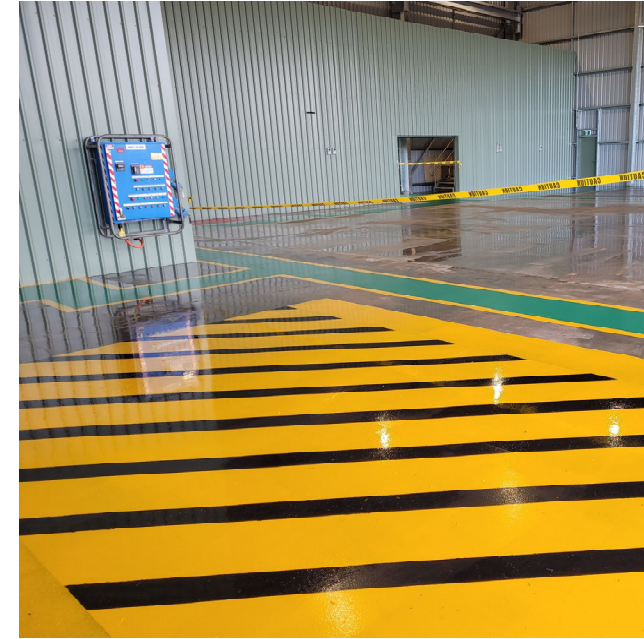
Surface workshop – commissioning near complete
